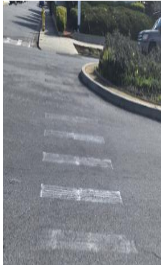
Figure 5-Faded Crosswalk on Woodrow St in the City of Santa Cruz
