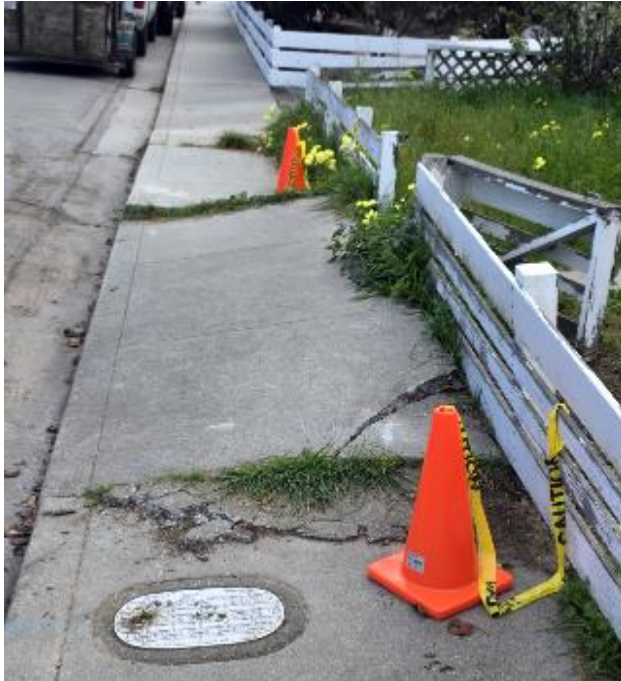
Figure 2- This sidewalk on John Street in the City of Santa Cruz is cracked and uplifted, causing a tripping hazard
